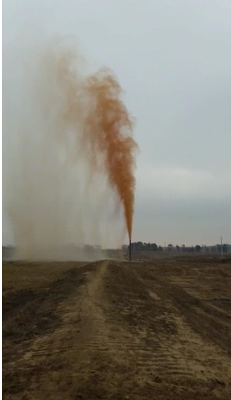
Figure 4 – Use of the "dynamic blowdown" method developed and implemented as part of SESC for cleaning the bypass piping of a linear valve assembly.
