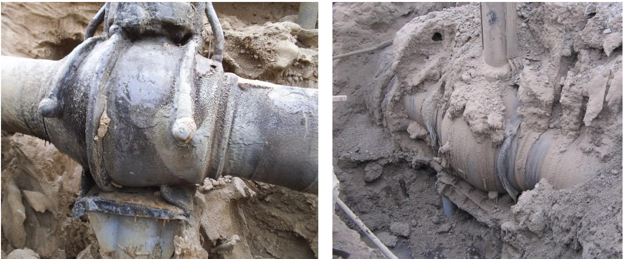
Figure 2 – Results of uncontrolled pipeline subsidence after soil thawing.
