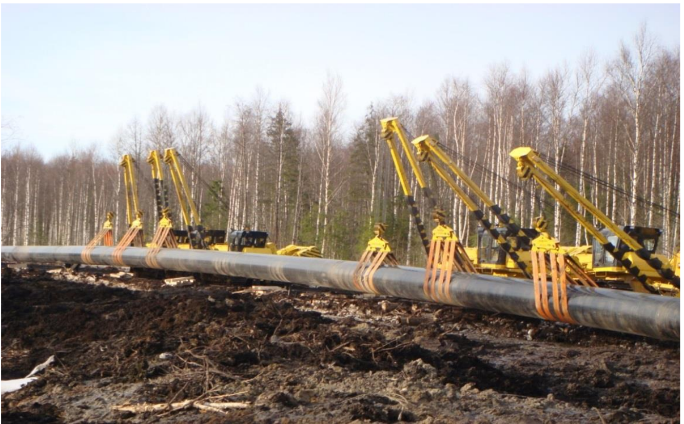
Figure 1 – Placement of pipelayers in groups due to the specifics of calculations performed at three suspension points.
